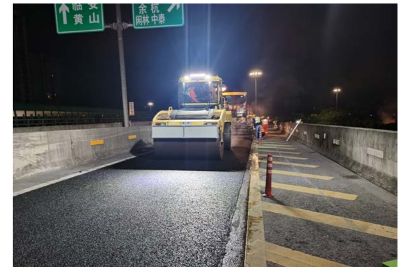
Nighttime traffic interruption and intensive construction site of the Hangzhou North Management Centre
